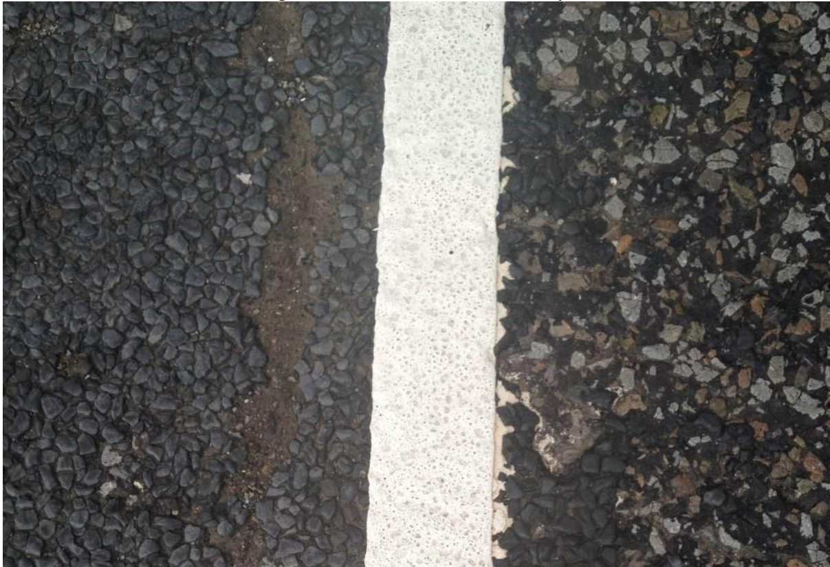
Figure C.2 Condition score 50 – close-up of profiled line designed for wet visibility
