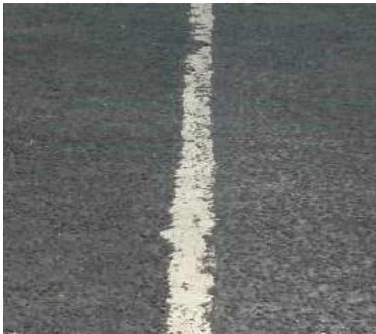
Figure C.8 Condition score 20 – close-up
